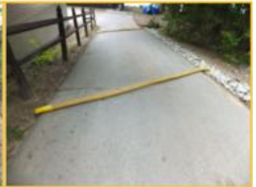
Firehose Diverter - In paved driveways, burying rubber and wood are not an option. Old firehose, or other durable material, can be filled with sand or stone and placed on an angle to divert stormwater. These have the added benefit of being movable.
